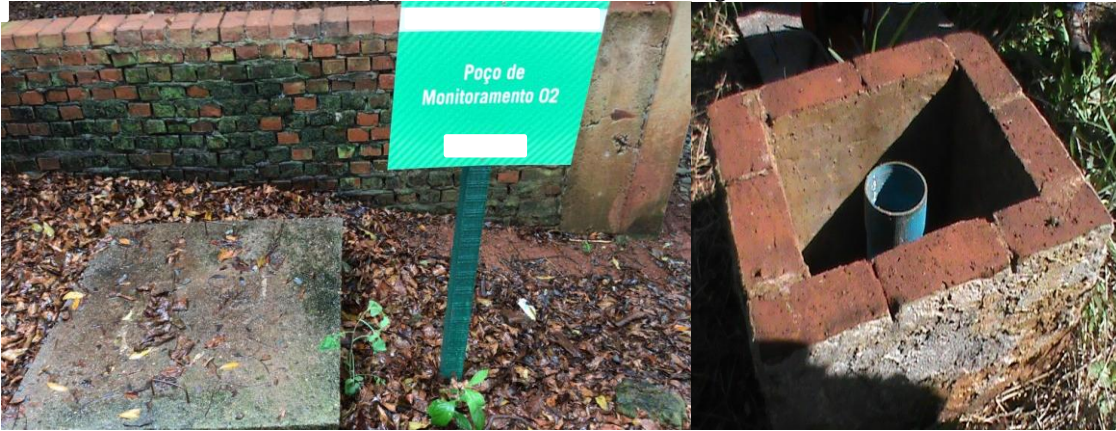
Figure 5 - Groundwater monitoring wells.
