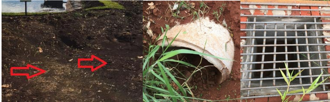
Figure 7 - Storm drainage system.
